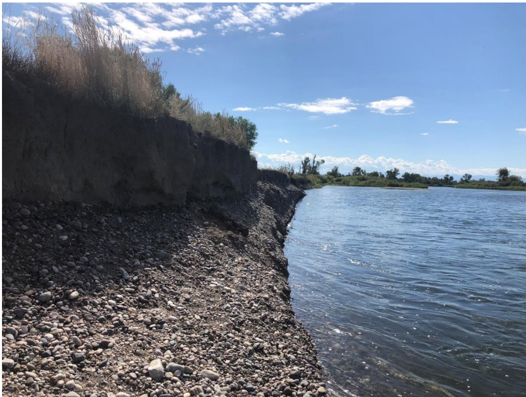
Figure 5. Photo showing sloughing, unstable banks and dangerous conditions for visitors looking upstream from the confluence.
